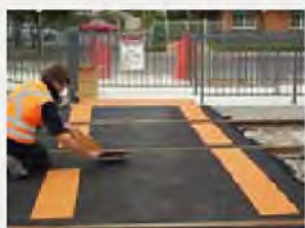
Important safety features at railway crossings
